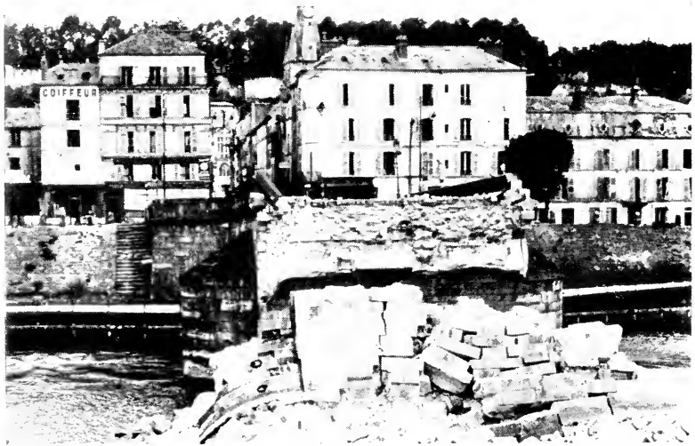
BRIDGE CROSSING MARNE RIVER IN CHATEAU-THIERRY DESTROYED BY GERMANS IN THEIR RETREAT FROM TOWN
